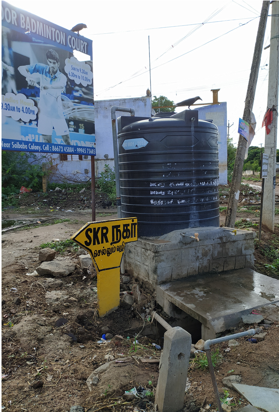
Fig 12: View of drinking water infrastructure in Koundampalayam ward. Source: GIZ India
