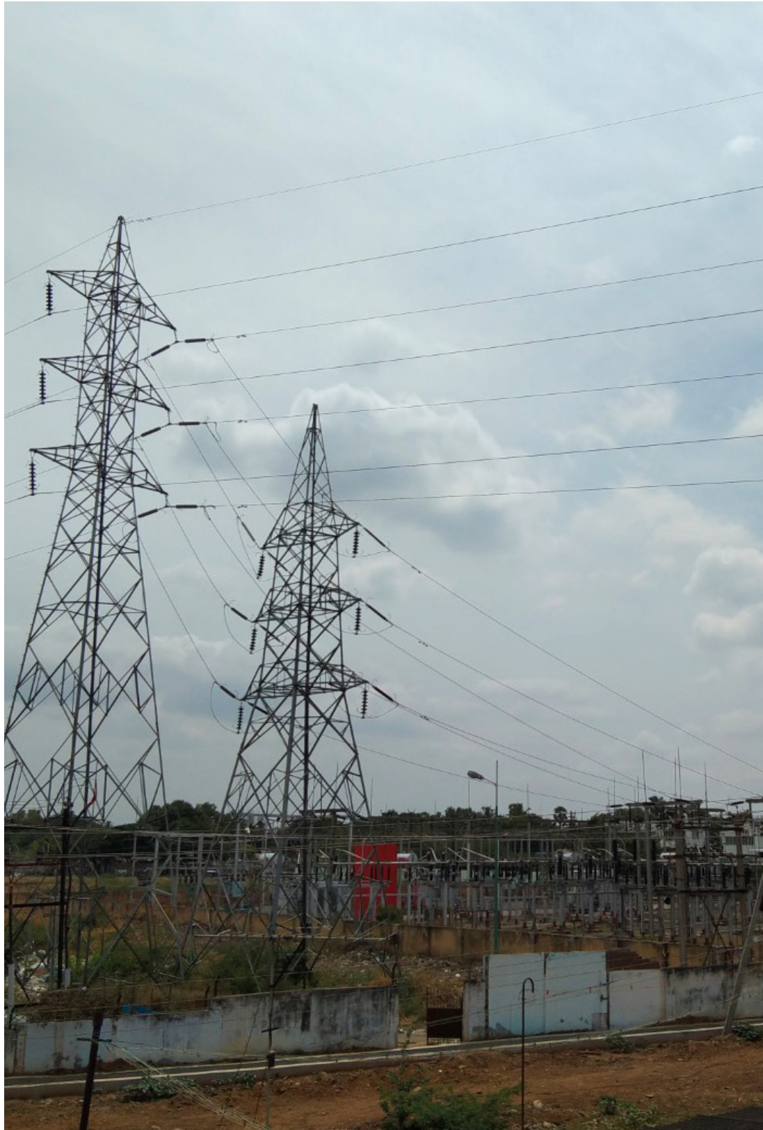
Fig 44: View of TNEB substation near Subsite C. Source: GIZ India
